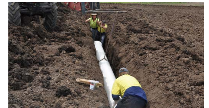
Figure 4.11 – Installation of underground piping for drip irrigation systems in tea tree plantations. Subsurface distribution supports efficient water use and reduces surface runoff.
