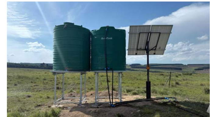
Figure 8.1. Solar-powered water storage infrastructure installed through Fair for Life premium allocations derived from TTO sales.
